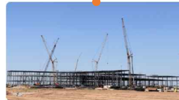
[LG ES Project in Queen Creek, AZ]
